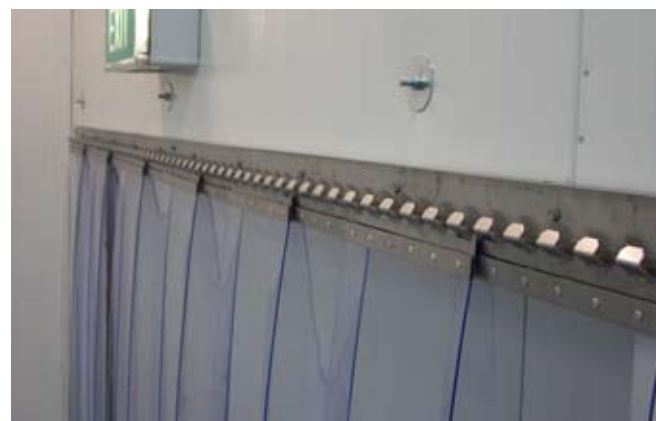
Note the sequence of hanging the PVC strips, ensure the correct strip overlap and cover.
