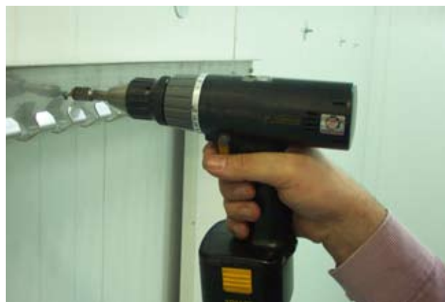
Fixing the headrail to the doorjamb using a battery powered drill and self drilling screws
